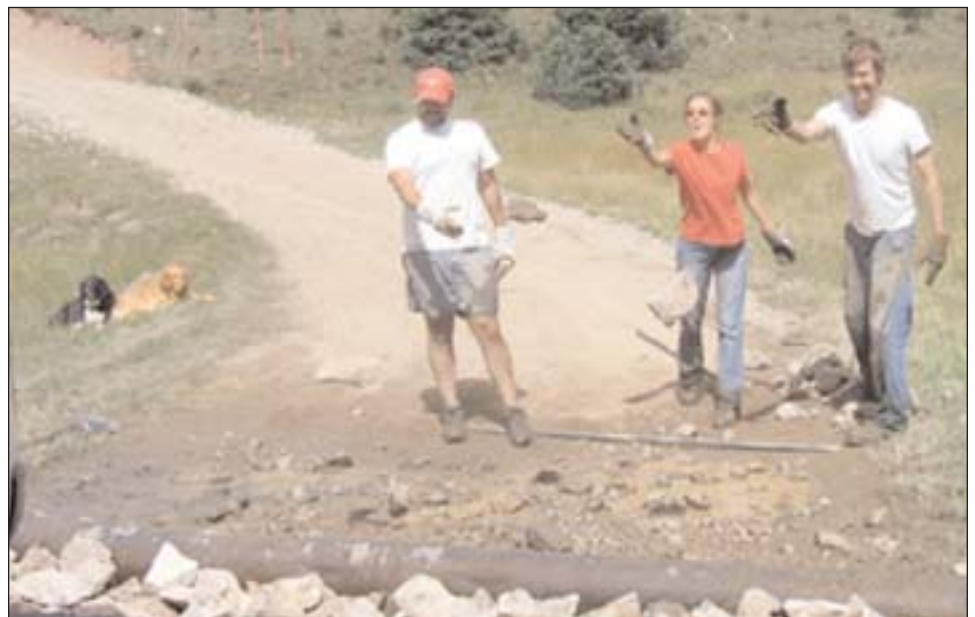
Scooby and Scout supervise Erik Schlenker-Goodrich, Western Environmental Law Center, and volunteers Lauren Kawas and Ethan Timm adding rocks to the French drain
